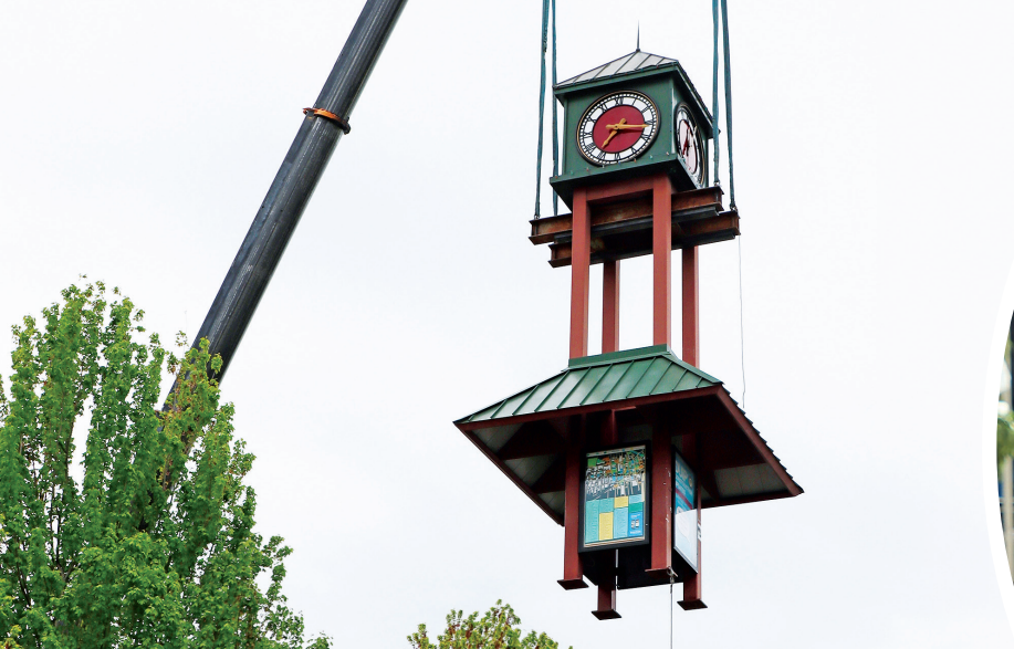
Construction on the Downtown Utility Improvement project necessitated the temporary relocation of the clock tower. The tower will return to its spot later this summer.
